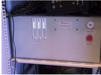
Figure 4: Autoscope Detector Rack Card interfaced with SCADA system
