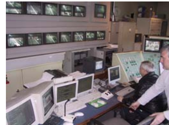
Figure 5: Clyde Tunnel control room
